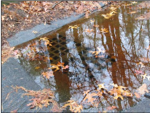
The catch basin at the White Pond public access boat launch quickly reached capacity, allowing untreated or minimally treated stormwater to flow directly down to the pond.
