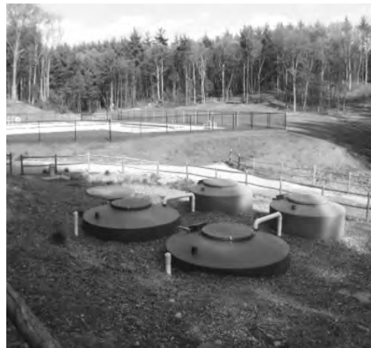
A closer view of the treatment tanks. The "tall" tanks are about 2 feet high. The wide tanks are between 5 and 6 feet in diameter. The fenced area is a swimming pool. The leaching field is under the nearby recreation fields.
